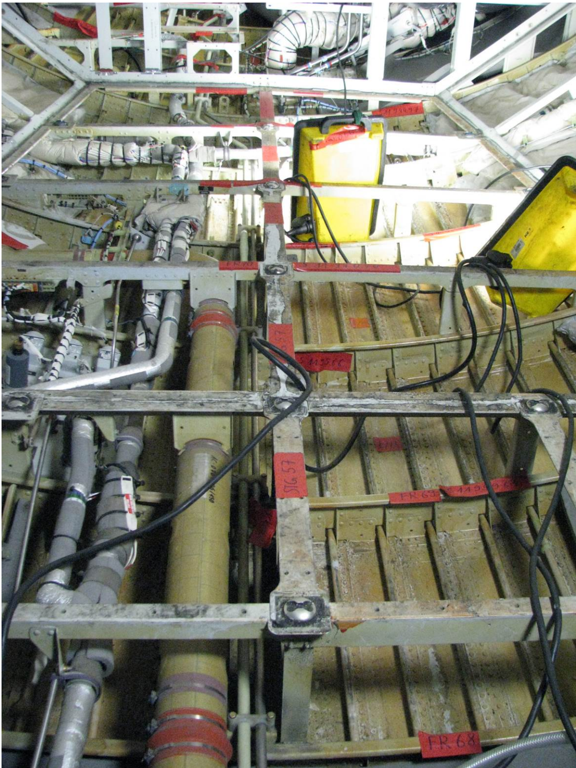
Damaged area inside the fuselage, in the foreground frame 68 (FR 68), in the middle stringer 57
