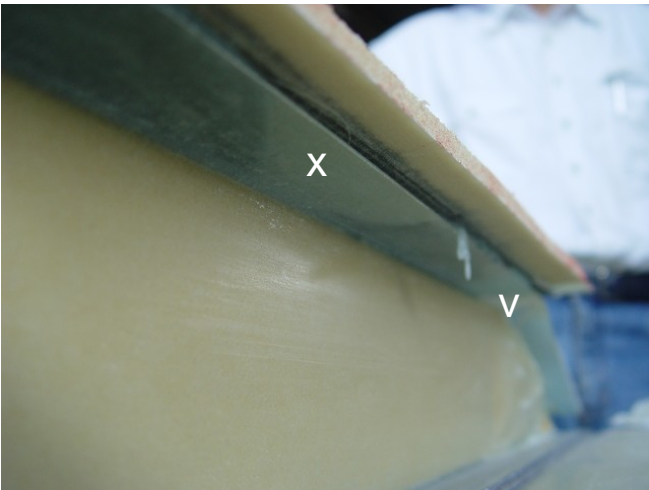
Picture 5: Flawed bonding (x) and excessive (v) adhesive
