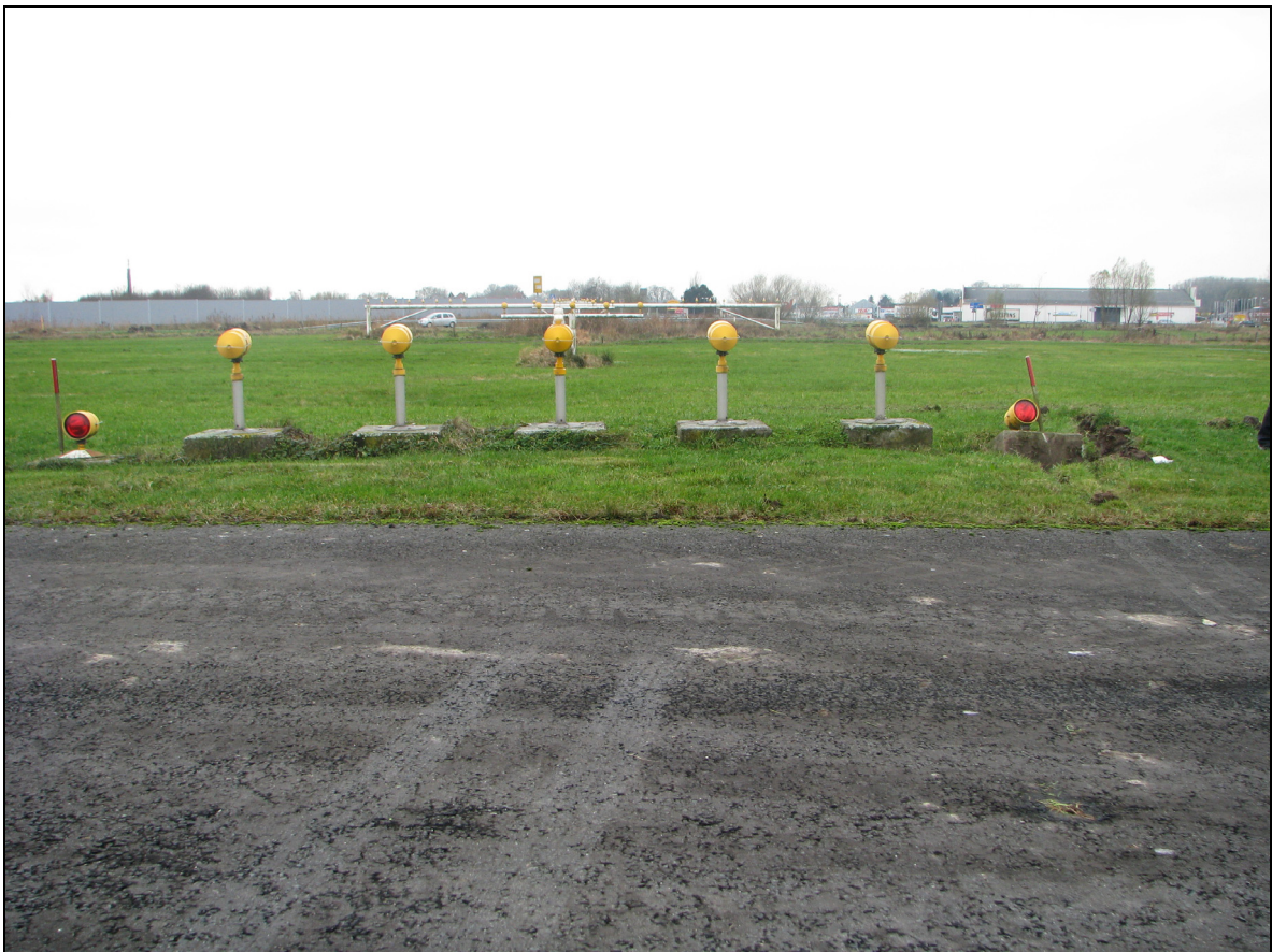
Runway lighting on concrete plinths
