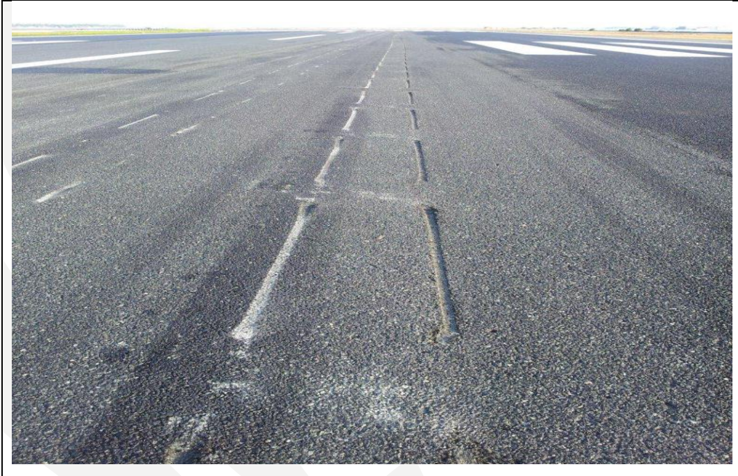
Photo 29. Damage on the runway surface.
