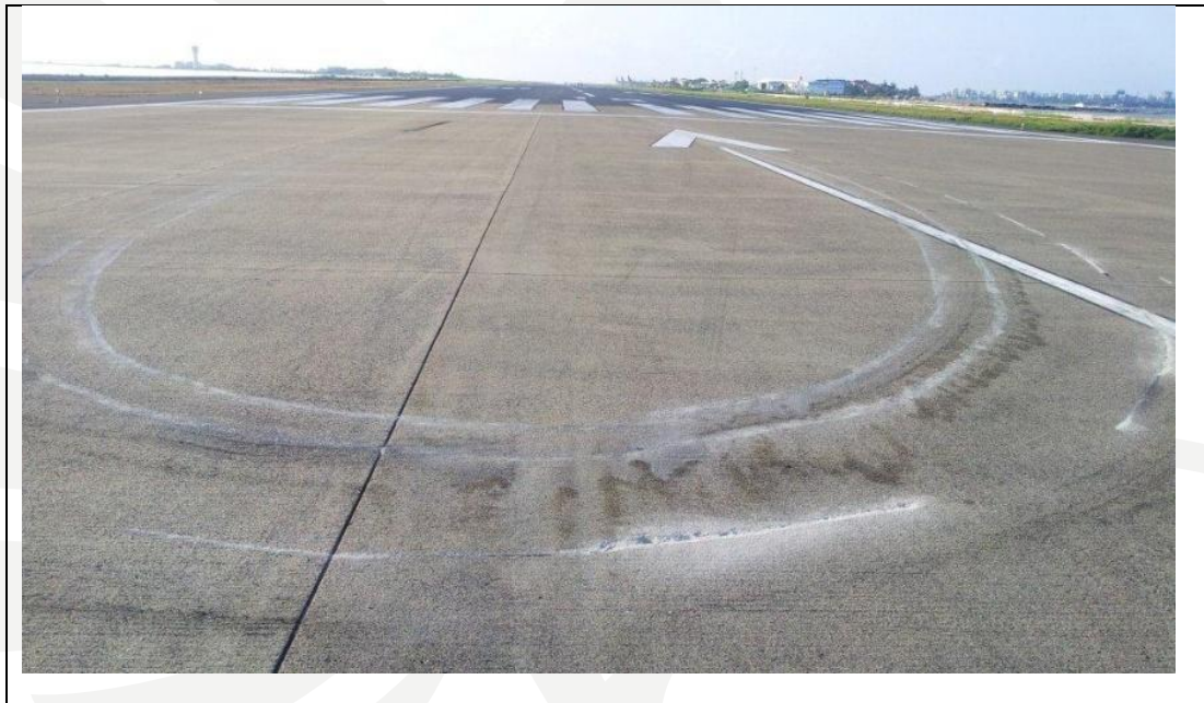
Photo 30. Runway 18 threshold area showing the damage on the runway surface.
