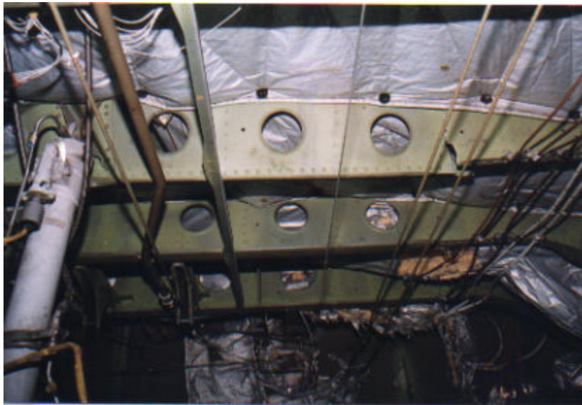
Photograph 4. Bend and Tear out on Upper Frame #43
