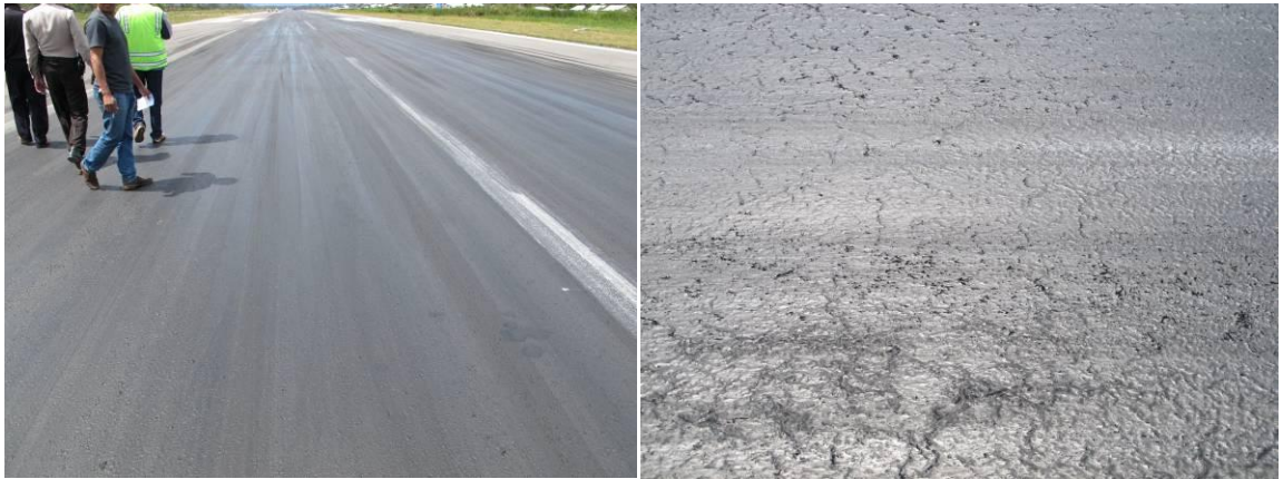
Figure 4: Rubber deposit on runway 15
