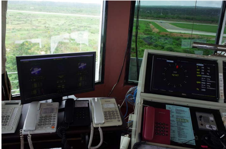
Figure 4: AWOS display (left) and Tower Set display (right)
