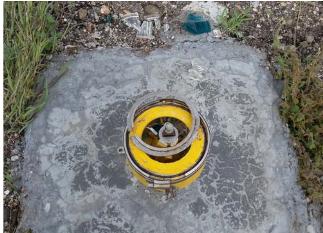
Figure 2: The broken runway light
