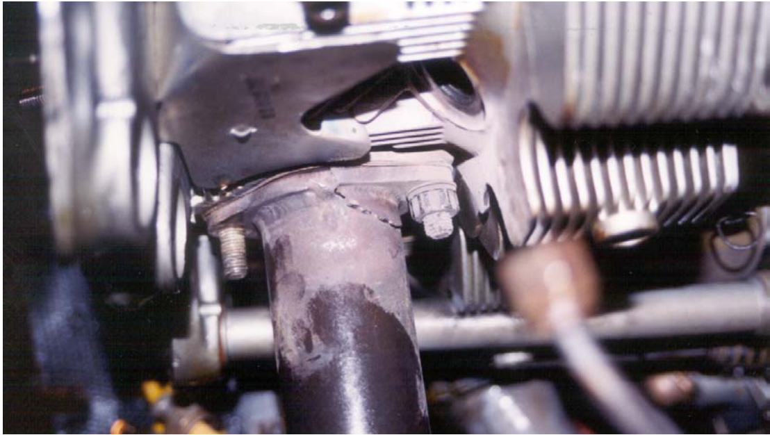
Cracked Exhaust Stub (as found on the engine – the missing nut was removed during the investigation) Fig. 3
